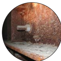
Rust and Corrosion
